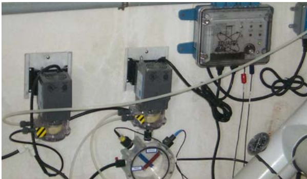
Figure 4-3: Liquid feeders controlled by an ORP unit
